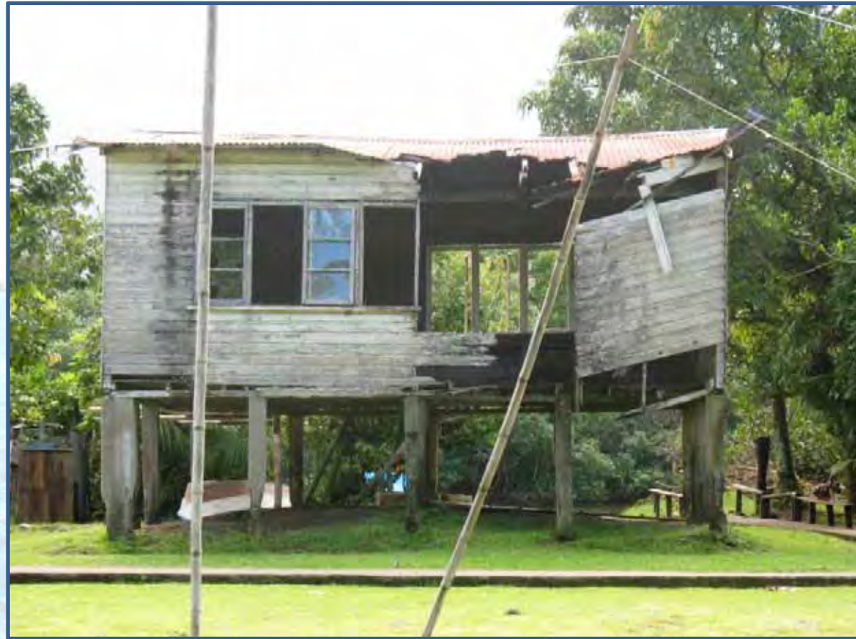
Muanaira Village, Rewa Delta, Fiji. 1990s adaptation to floods involved raising house on piles (Shalini Lata photo)
