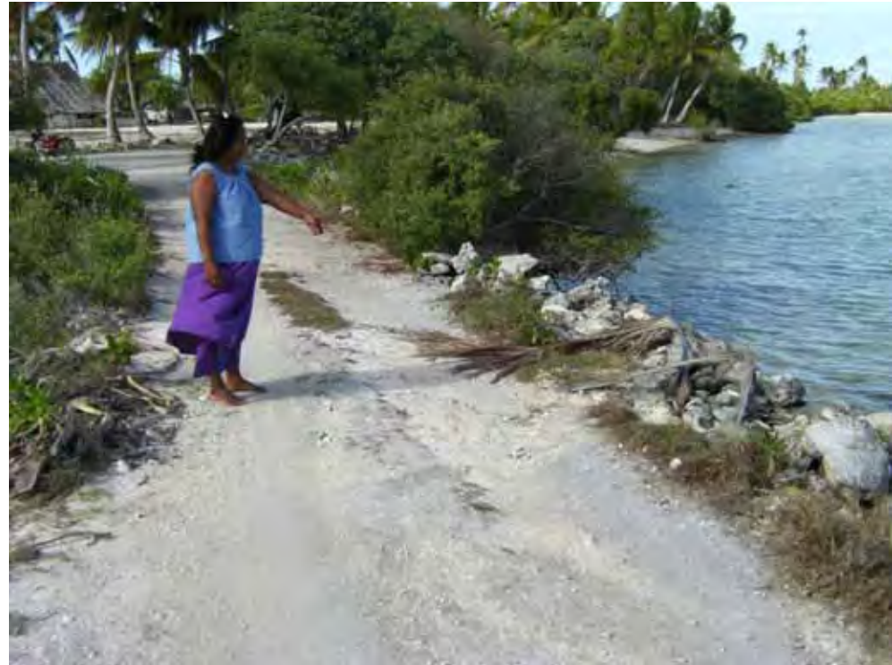
Eroding shoreline and seawall, Butaritari, Kiribati
